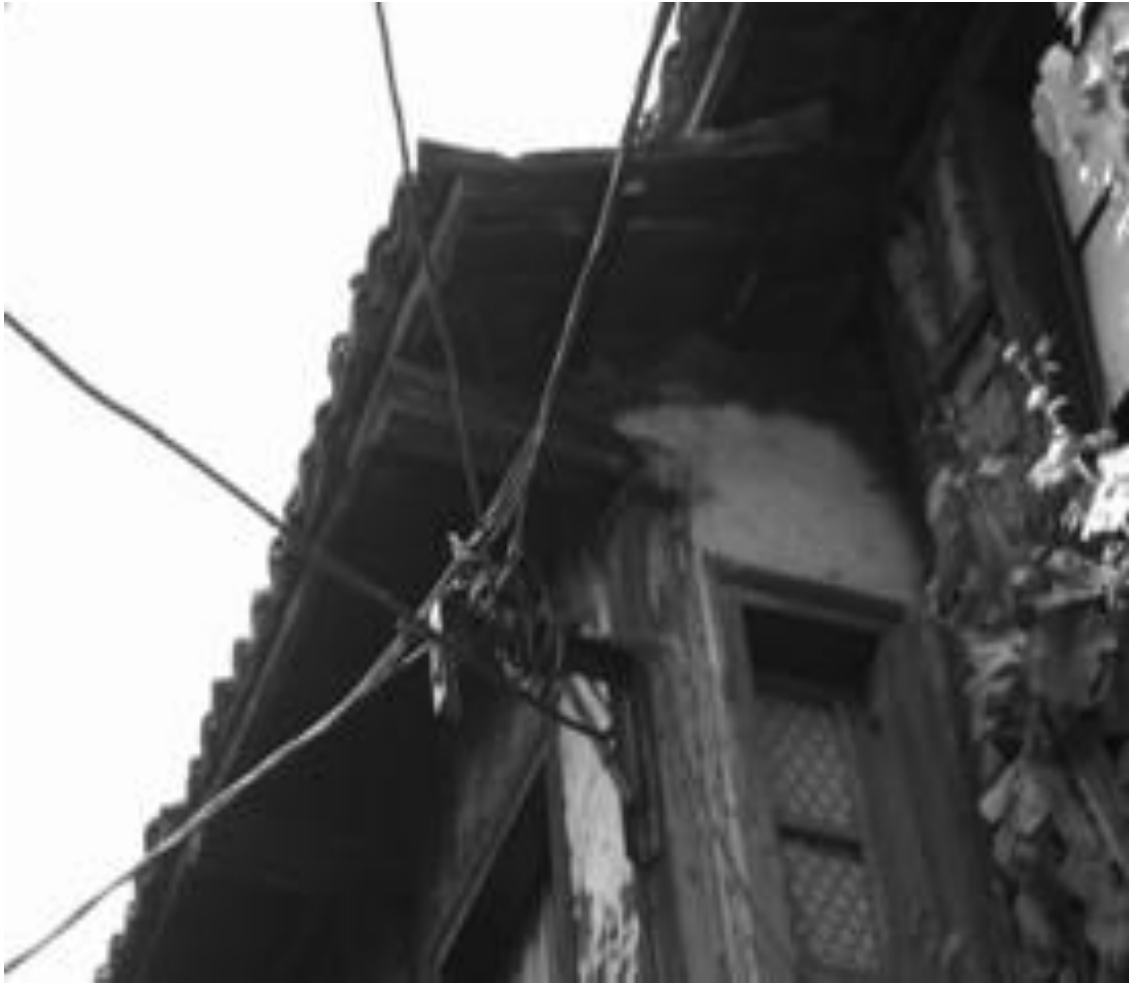
Figure 6. Dangerous Electric Wires
